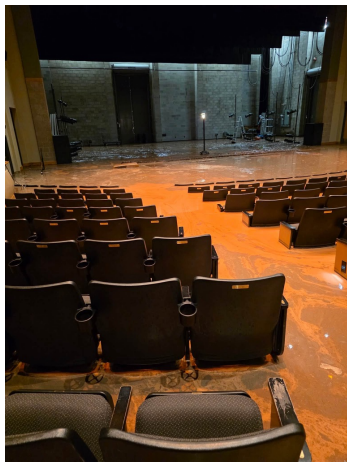
Palm Theater in Telluride filled with mud on July 17. From Telluride Fire Protection District
